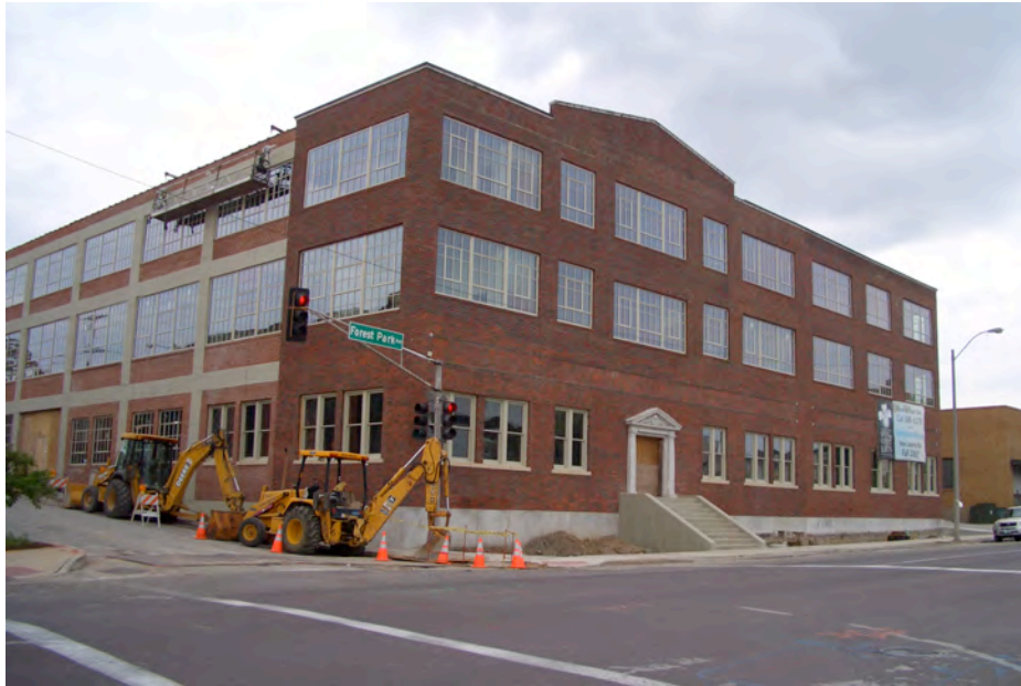
Lofts Apartments Being Renovated On The West Side of 3663 Forest Park Avenue
